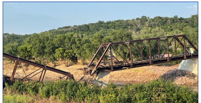
COLLAPSED BRIDGE. This nationally-televised picture of the collapsed railroad bridge in Sioux City shows the destructive force of the raging Big Sioux River during floods in June.
